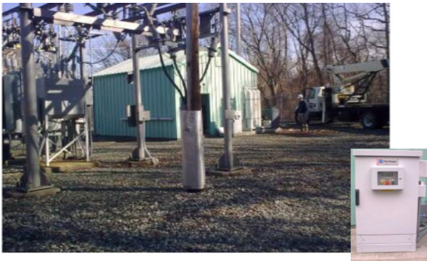
Figure 16 - National Grid USA- Barrington Site
